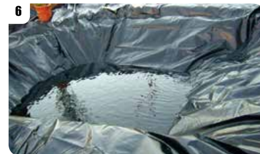
6 Weigh liner edges down then smooth away folds as water starts to fill the pond.
