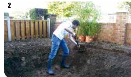
2 Finishing the dig by hand - digging out shelves and smoothing the surface. Get rid of as many stones as you can.
