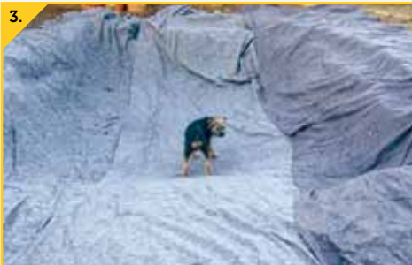
3. Due to the very stony nature of the ground we chose to upgrade to Fleece Underlay (Dog optional!)
