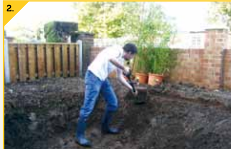
2. Finishing the dig by hand - digging out shelves and smoothing the surface. Get rid of as many stones as you can.
